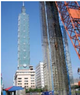
Taipei Rapid Transit System (Metro)
