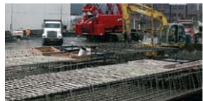
Big Pipe C50 Portland, Oregon USA
