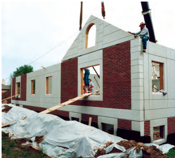
Fig. 13. Erection of the triangular sandwich wall panel. Note the variable opening configurations in rectangular and triangular panels.
