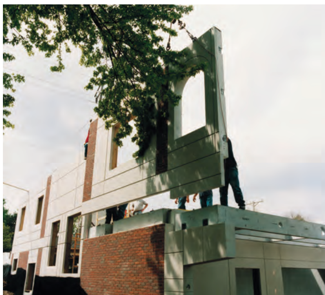
Fig. 15. Setting an exterior wall panel in place. Note the attractive finish treatment of these panels, emulating brick and masonry construction.
