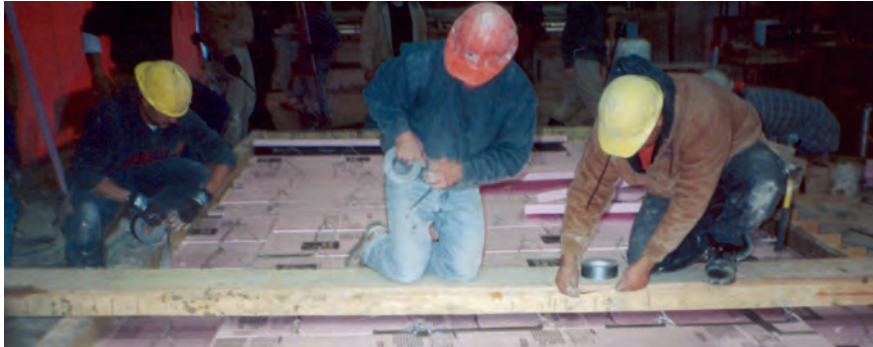
Fig. 12. Workers installing the insulation foam for the middle layer of the rectangular sandwich wall panel.
