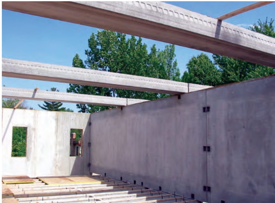
Fig. 19. Roof beams in place between partition wall and exterior wall of home.
