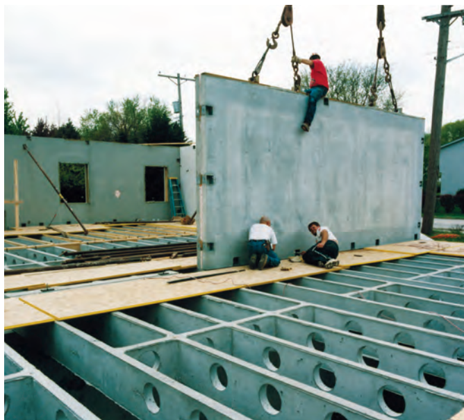
Fig. 14. Setting an interior wall panel in place. Note the openings in the floor beams in the foreground.
