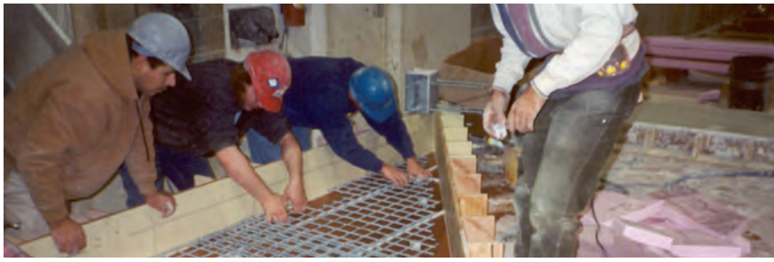
Fig. 11. Workers installing the welded wire reinforcement for the first layer of the triangular sandwich wall panel.
