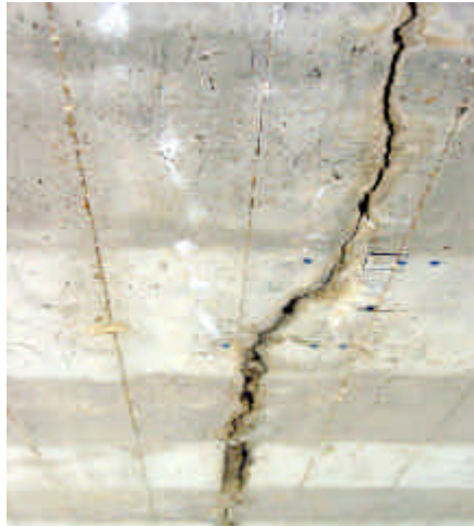
Figure 3 – Soffit Slab Longitudinal Crack
