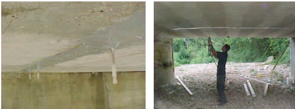
a) Crack Sealed Previous to Injection b) Crack Injection under the Bridge
