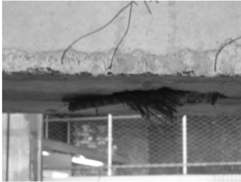
Fig. 7 Detail of the rupture of the CFRP bar in Beam C.2
