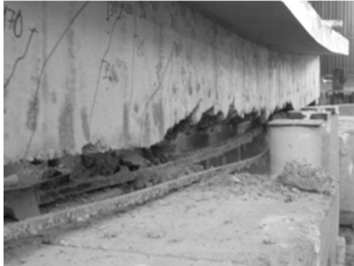
Fig. 5 Detail of the CFRP strips strengthening peeling off - Beam B.2
