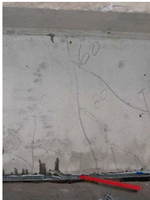
Fig. 8 Detail of the debonding of the CFRP laminate - Beam E.2
