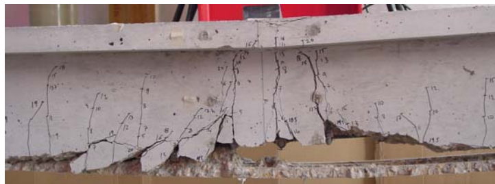
Figure 8 – Debonding failure of beam B4 strengthened with five NSM thermoplastic GFRP strips
