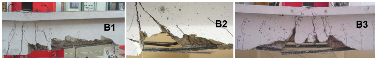
Figure 4 – Failure of beams strengthened with NSM CFRP rebar and strips type 1 and type 2
