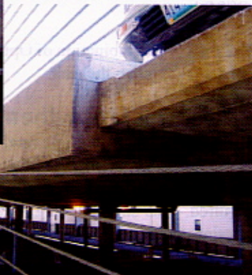
Fig. 5: Cracking on slab edge shown before and after repair
