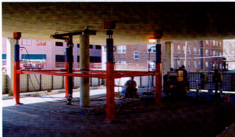
Fig. 1: Load testing of slab using hydraulic jacks and steel frame to apply the loads. Note the computers acquiring data
