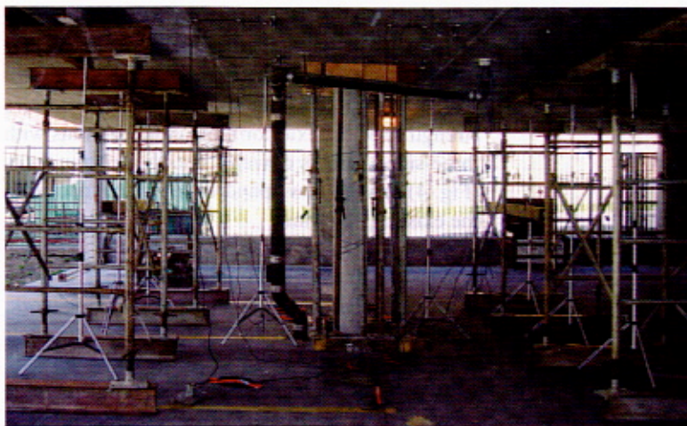
Fig. 2: Underside of test slab showing sensors during load test of Option 2. Shoring was used as a safety measure (it was not in contact with the slab bottom)
