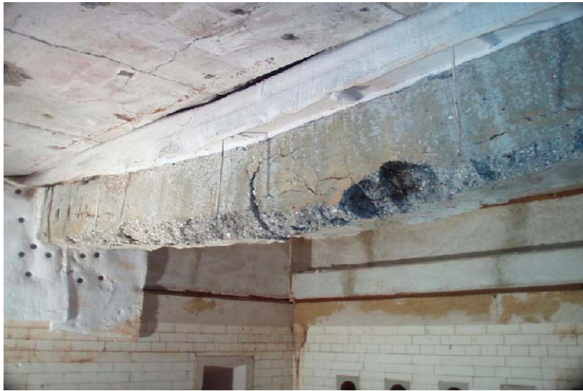
Fig 4 Rupture at the mid centre of the concrete in beam 1 after fire test
