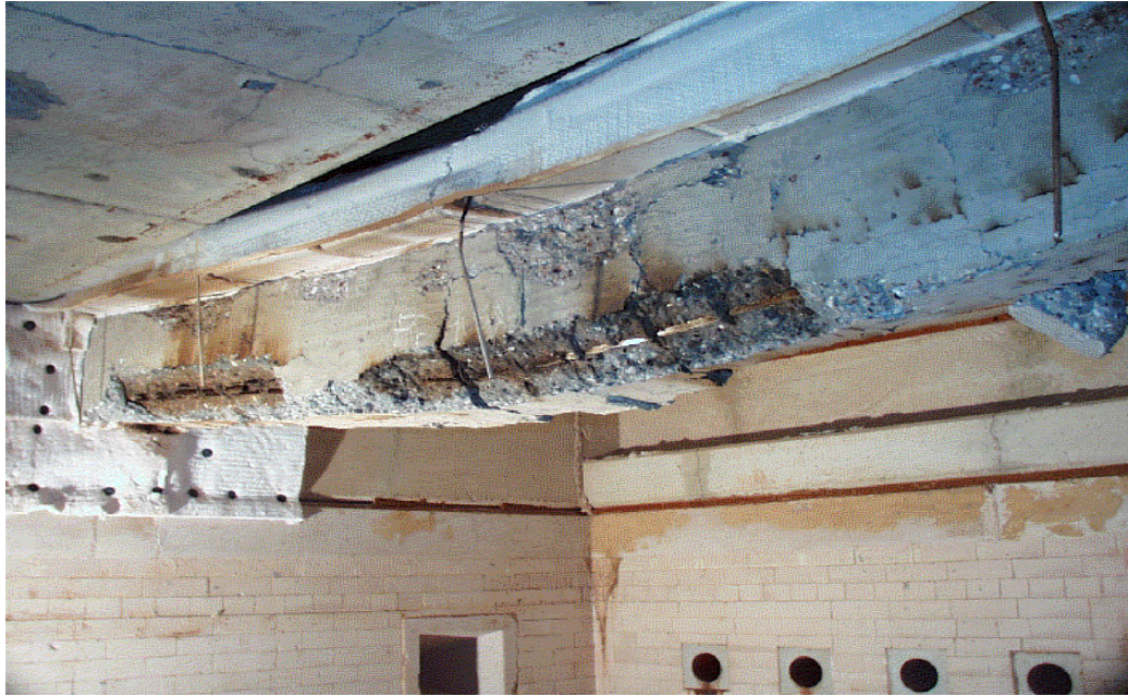
Fig 5 Failure of beam 2 after fire test inside the furnace shows some flexural cracks and rupture in the main reinforcement
