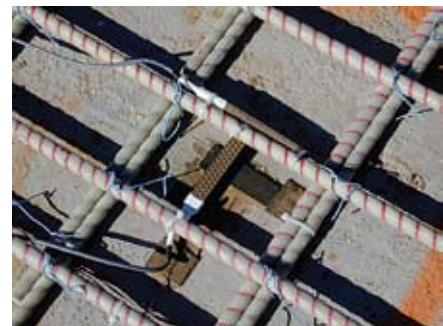
Concrete strain gauge for long term monitoring.
