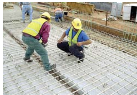
Traditional rebar chairs are used but with greater frequency. i.e. 2/3 rd s spacing used with steel.
