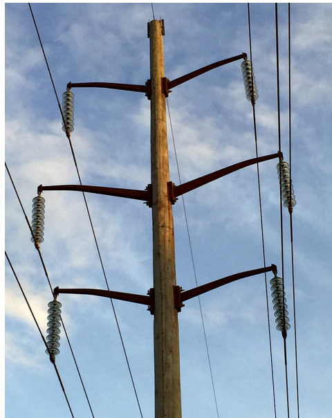
Weathering steel davits on round wood pole
