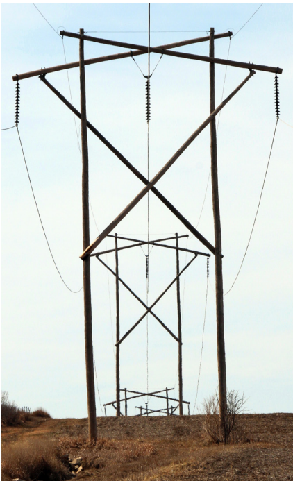
Aging spar-arm structure, shorter service life due to eccentricities of loads and sub-standard framing.
