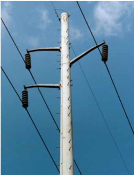
Galvanized steel davits on spun concrete pole
